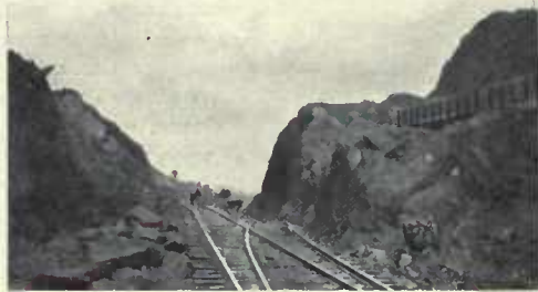
In the Trap Rock—A section of the Canal at Bas Obispo, where the excavation is down to the stratum which must be drilled and blasted.
