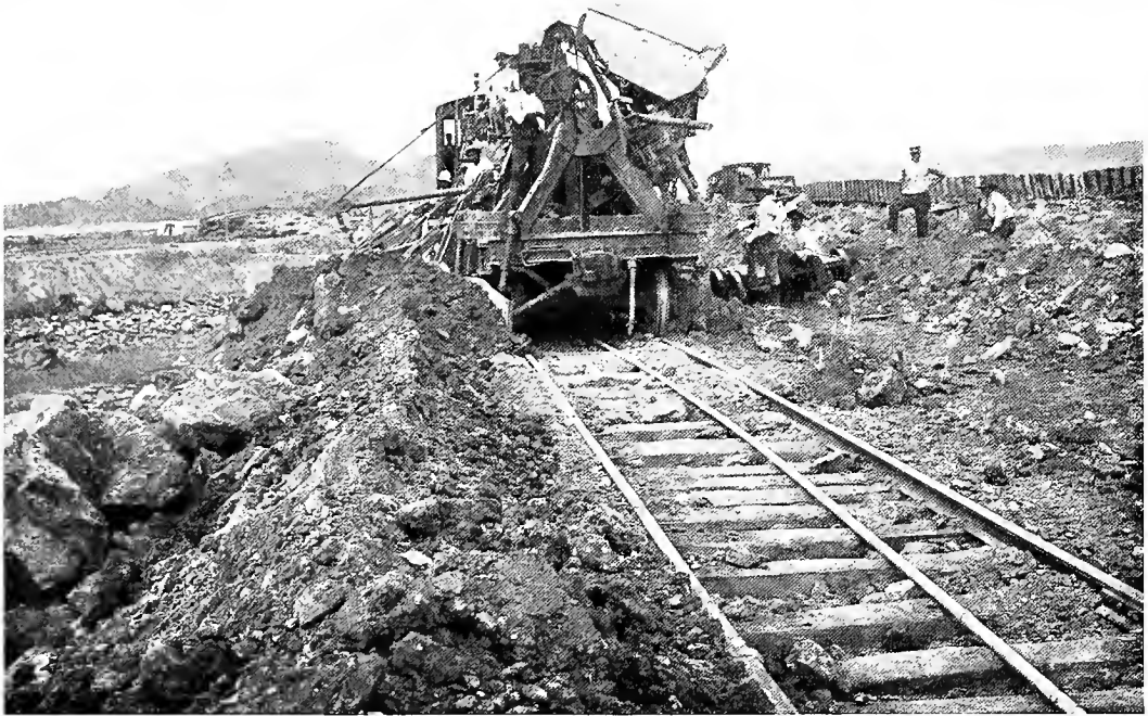
1. Side view of dirt spreaders at work on the dumps. 2. Front view of same.
