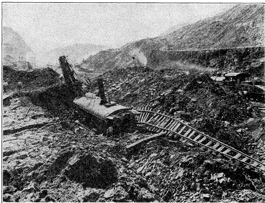
FIG. 63.—EAST CULEBRA SLIDE SHOWING UPHEAVED MATERIAL BETWEEN STATIONS 1746 AND 1758, FACING SOUTH, FEBRUARY 6, 1913
